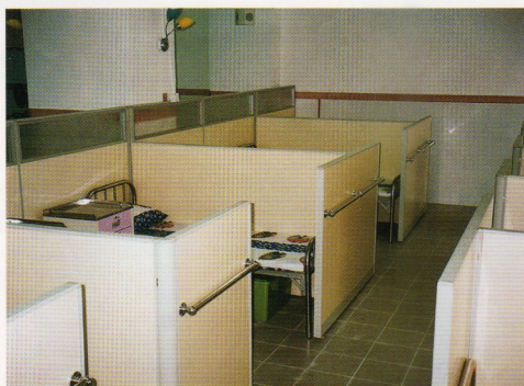
護老院防火板面屏風間格及不銹鋼床
